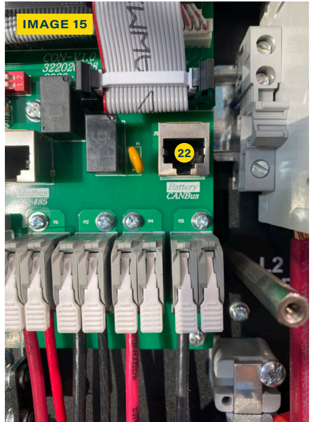
22 CANBUS PORT ON SOL-ARK INVERTER
