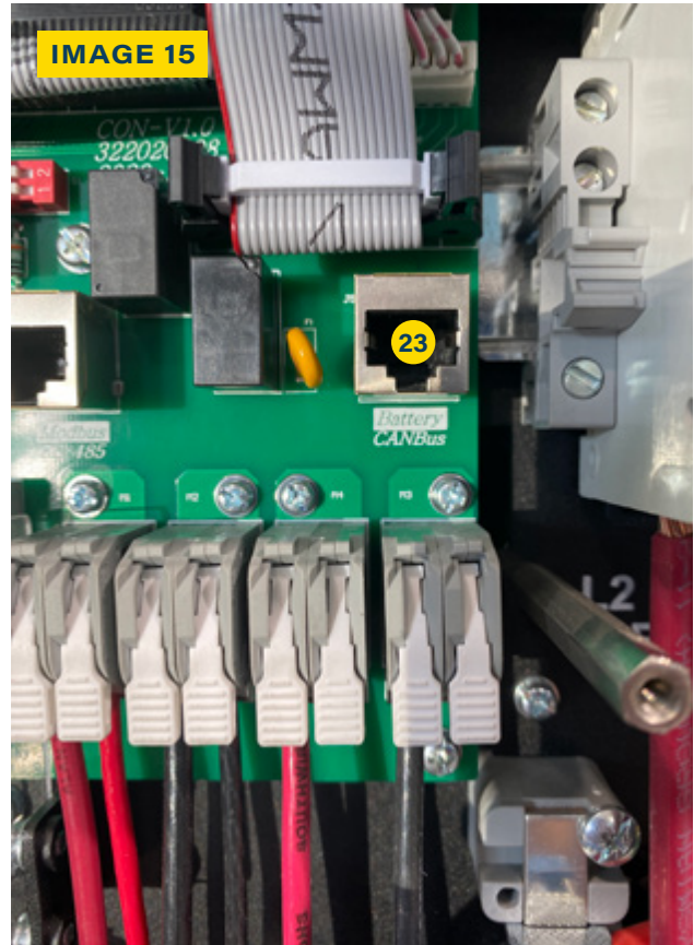
23 CANBUS PORT ON SOL-ARK INVERTER.
